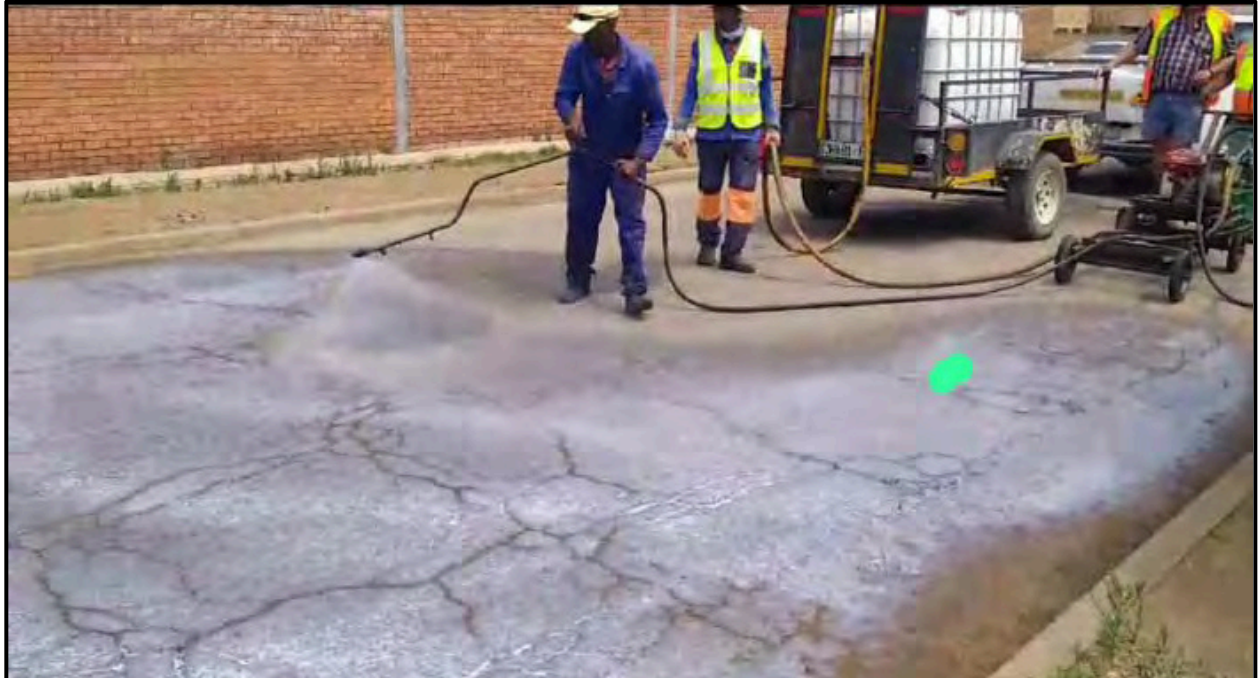
Figure 85 Application of a NPNS clear seal from a flow-bin on the back of a trailer
